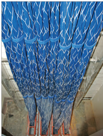
Cabling pathways and spaces are limited for older buildings like Pond Laboratory. A vertical closet system was installed to accommodate the cabling.
